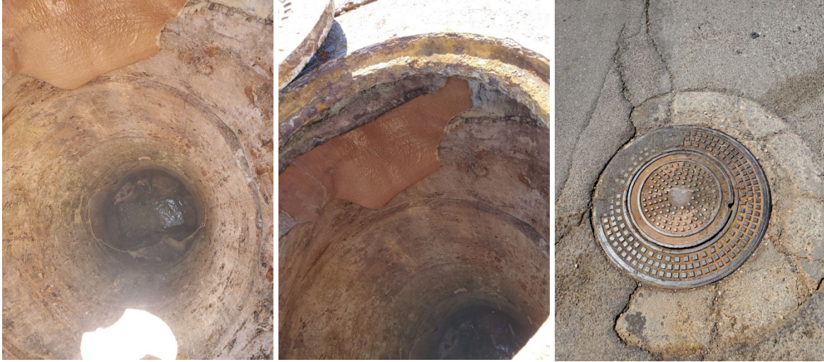
Depth- 16ft Complete liner failure, disrupting flow. Collar and concrete deteriorating.
