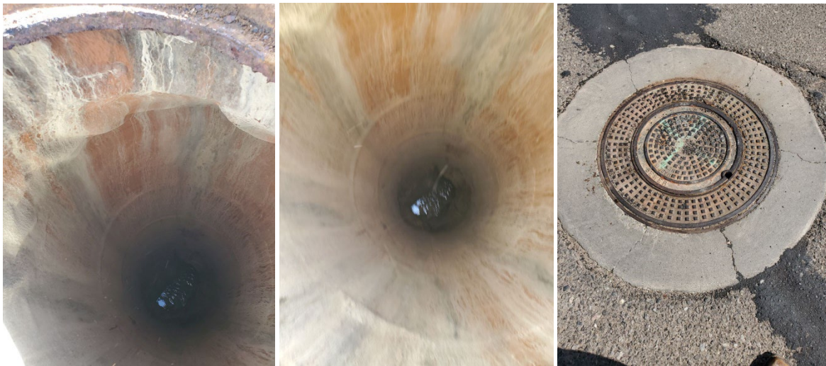
Depth- 21ft Bubbling in liner, bottom of liner is gone
