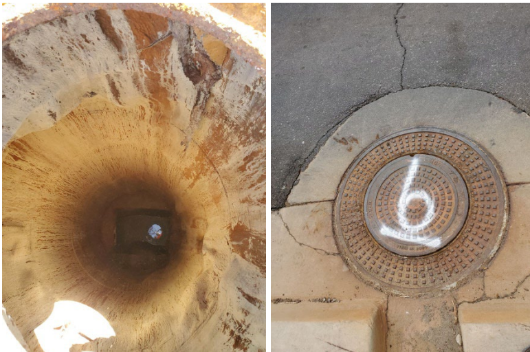
Depth- 17ft Liner bubbling and deteriorating
