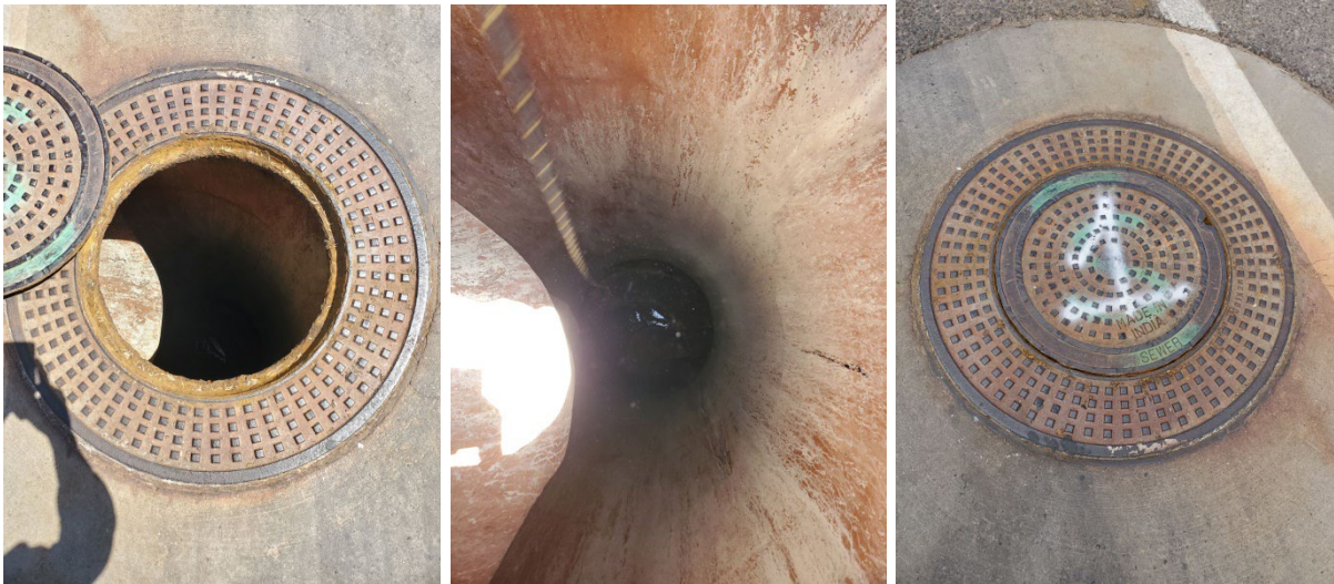
Depth- 17ft Bubbling in liner/ bottom liner is gone and disrupting flow
