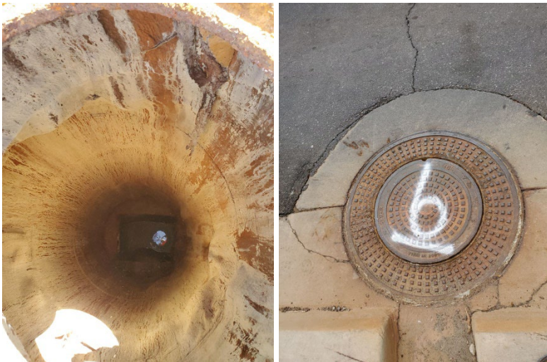
Depth- 17ft Liner bubbling and deteriorating
