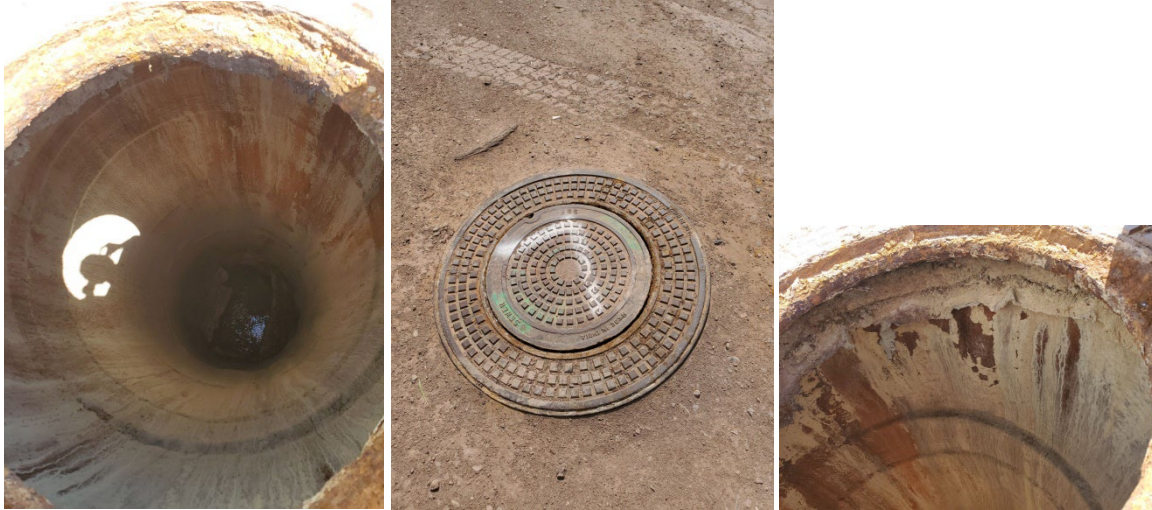
Depth- 20ft Bottom of liner is gone, collar is deteriorating
