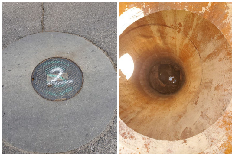
Depth- 17ft Bottom of liner is gone and disrupting flow
