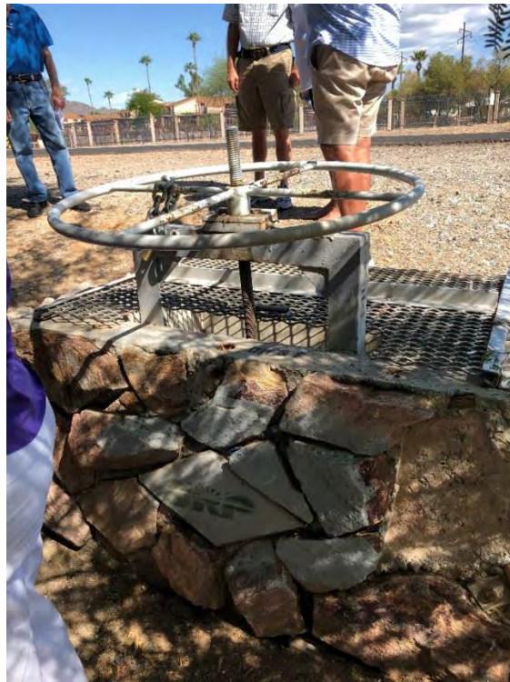
Photo 5-2: Weir Box on Underground Irrigation Line delivering Water to a Private Canal
